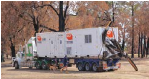
The new ablutions and office blocks arriving at the Bridgetown Golf Club.
